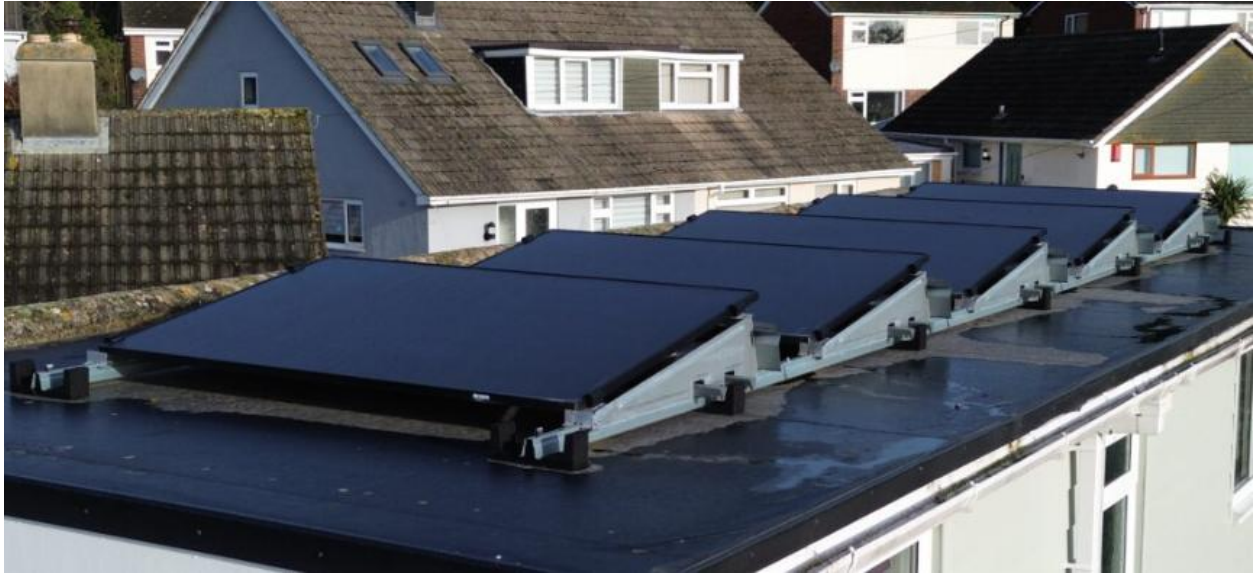
Panels on a flat roof without a parapet, mounted in an organized pattern, aligned parallel to with the edges of the roof.
