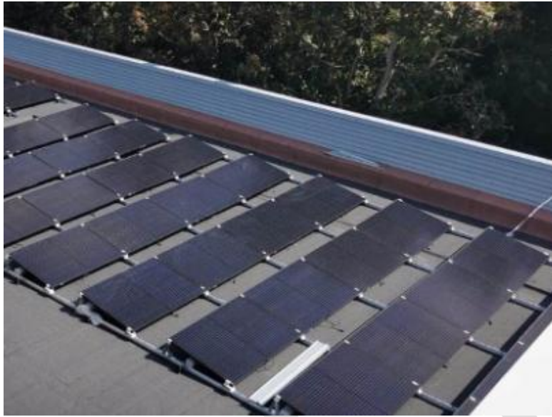
Panels mounted on a flat roof below parapet height.
