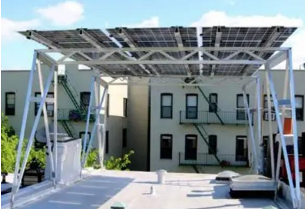
Panels on a flat roof with an obtrusive mounting design.
