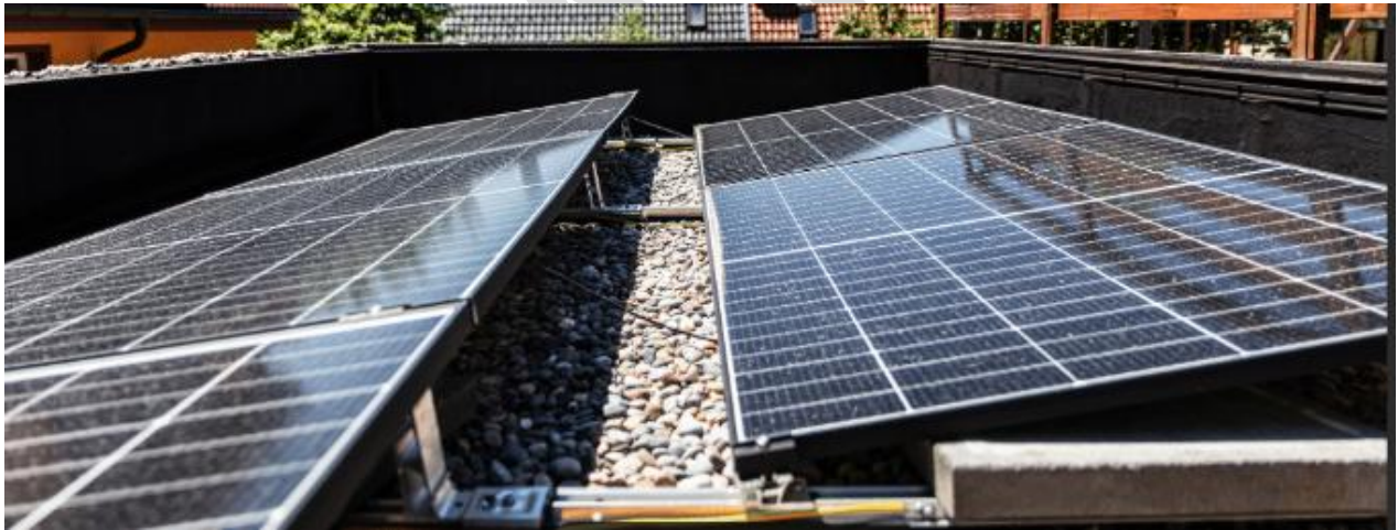
Panels mounted on a flat roof below parapet height.
