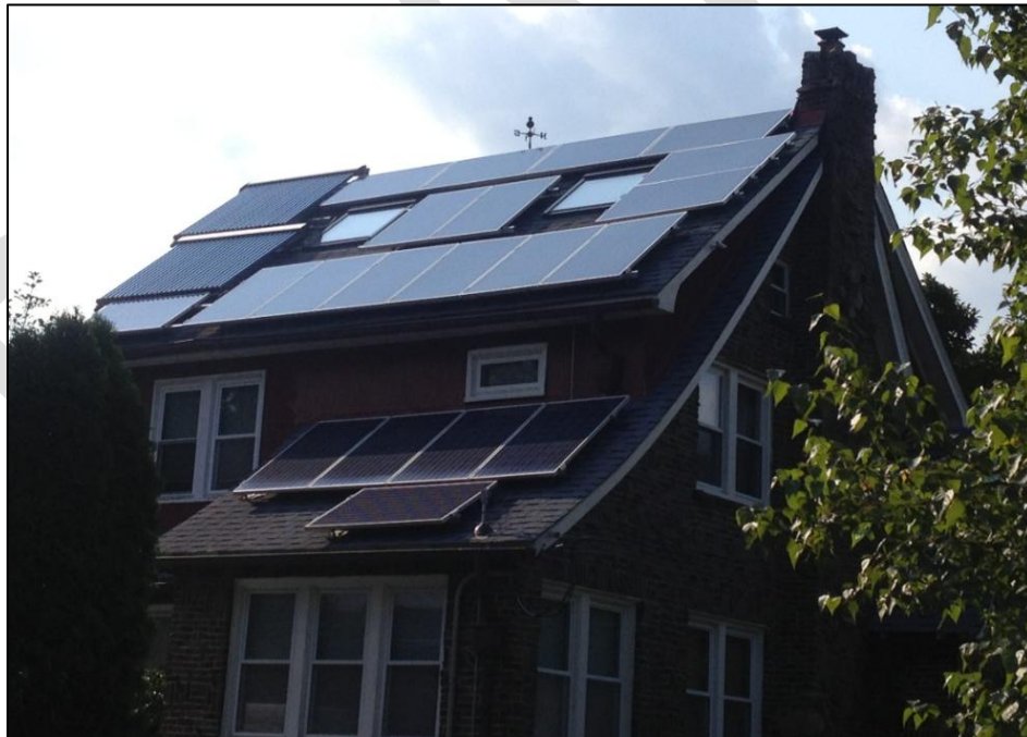
Panels with multiple sizes, colors and orientations on multiple roofs.
