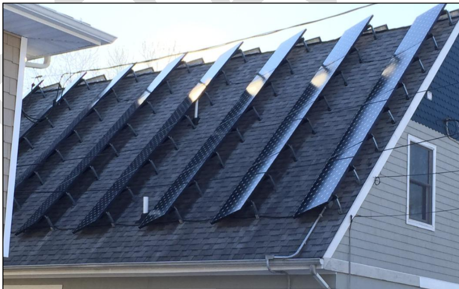
Panels mounted more than 6" from the roof plane and not mounted parallel to the slope of the roof plane and not flush with the roof.
